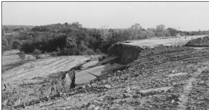
Landslide in westbound lanes of I-70 near New Concord, Muskingum County, 1986.
